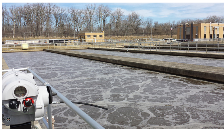
Under the sequenced pulsed aeration mode of operation, the aeration system now runs at lower DO levels, reducing energy use
