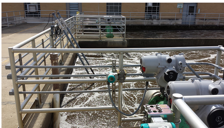
To support real-time monitoring and control, YSI IQ SensorNet sensors were installed in the basins
